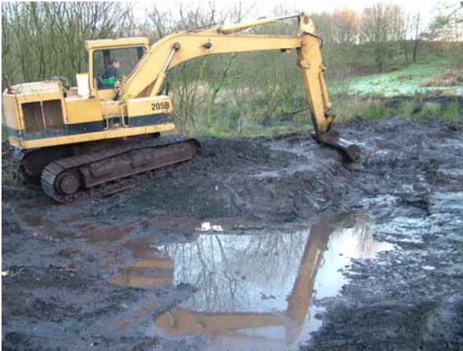
Pond creation underway in Blackburn, funded by the ARG UK 100% Fund. Photo by David Orchard
